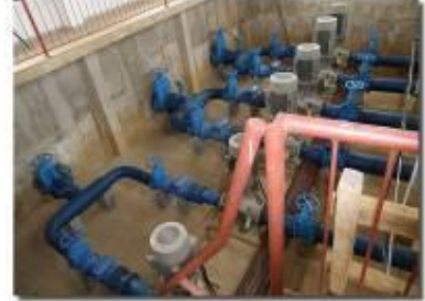
Impressive pumping station at Manyonyo. Some minor issues with debris / silt entering the foot valves
