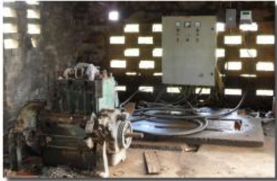
Old and new: the old diesel pump at Buleya replaced with an electrical one.
