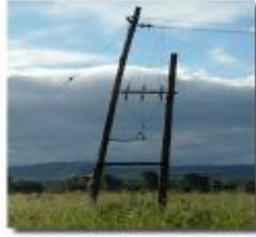
Temporary setback: ZESCO removed transformers recently at Sinazongwe and Nzenga
